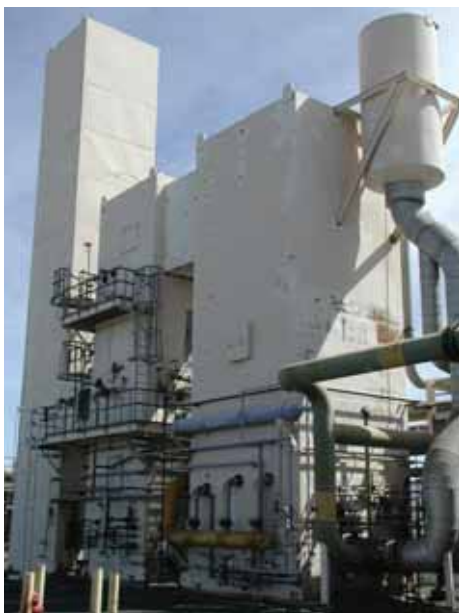
500-ton-per-day, 1981 cryogenic oxygen plant with reversing exchangers. Credit: Nils Tellier
